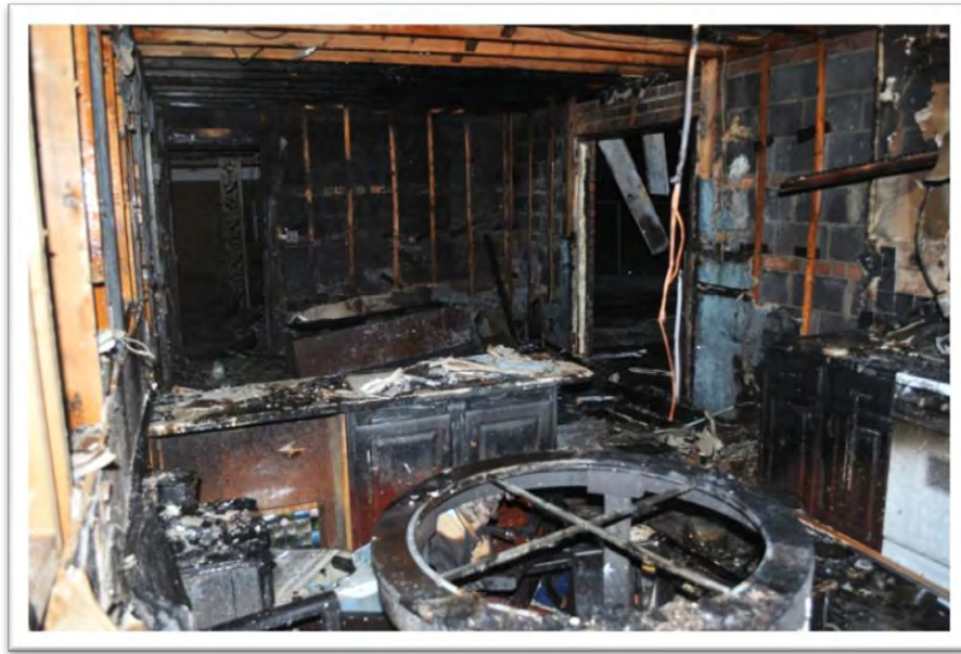
Figure 9: Kitchen area where injured fire fighters received burns. Note the hanging wire from the ceiling fan.
