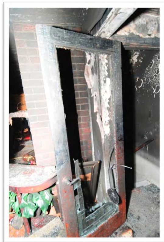
Figure 11: Door to the basement steps that were misidentified as the front door by the injured fire fighter.
